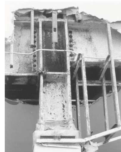
Fig. 1-3. Plastic hinging at top of column (Hall, 1995)
