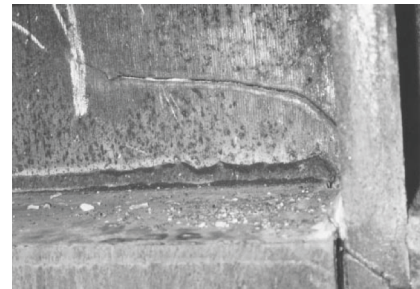
Fig. 1-2. Cracks through column flange and extending into web (Hall, 1995)
